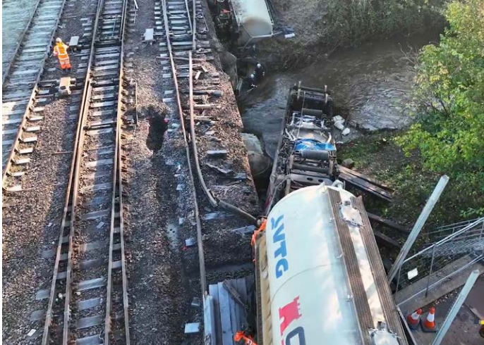
Upturned wagons in the River Eden and damage to tracks, bridge and formation. Photo: Network Rail
